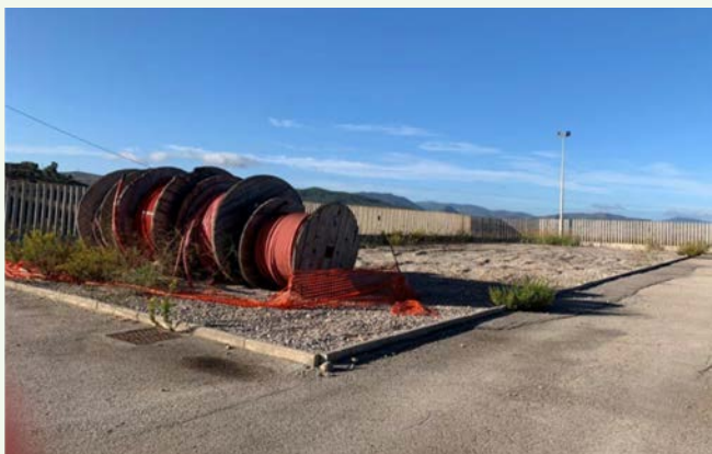
Installation area in the substation
